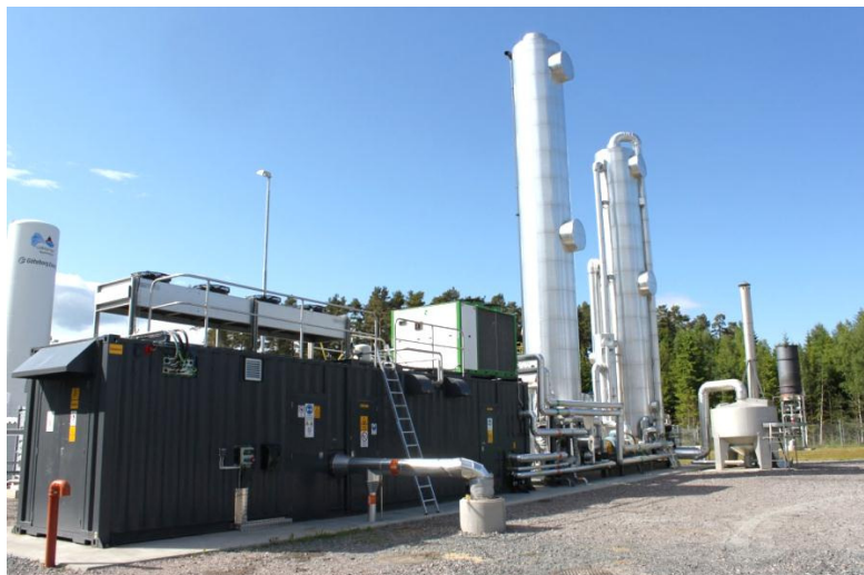
Figure 42: Water scrubber upgrading plant of Swedish Biogas International at Lidköping, Sweden (Source: Rutz)
