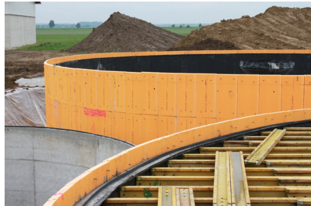
Figure 7: Insulation (orange panels) of digesters in Reichenkirchen, Germany (Source: Rutz)
