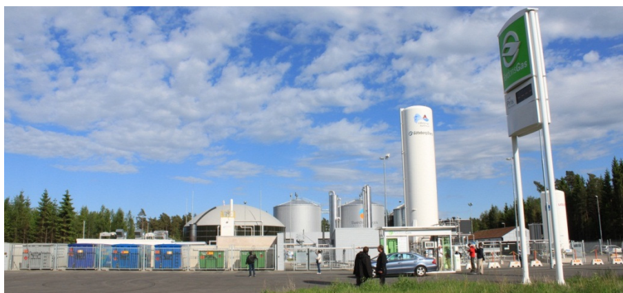
Figure 44: Biogas plant of Swedish Biogas International producing LBG in Lidköping, Sweden (Source: Rutz)
