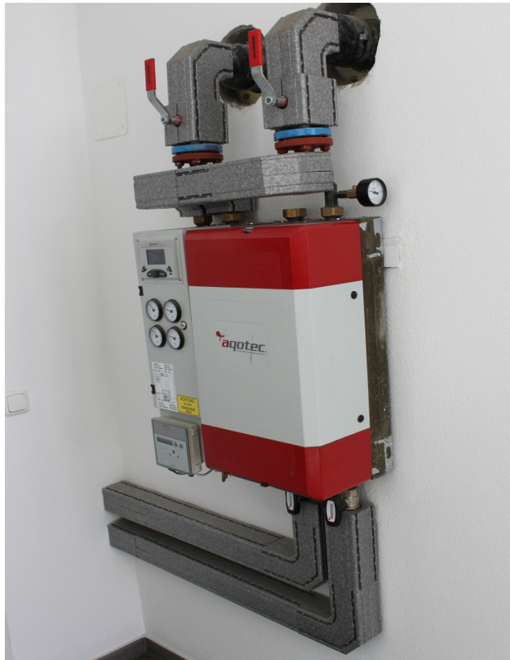
Figure 11: Connection equipment (including a heat exchanger) of an end consumer connected to a district heating system in Achenal, Germany (Source: Rutz)
