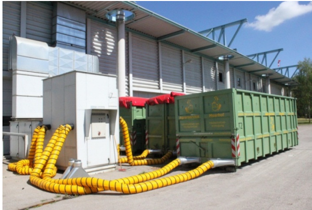
Figure 27: Container and air heating pipes for wood chip drying at a biogas plant in Munich, Germany (Source: Rutz)
