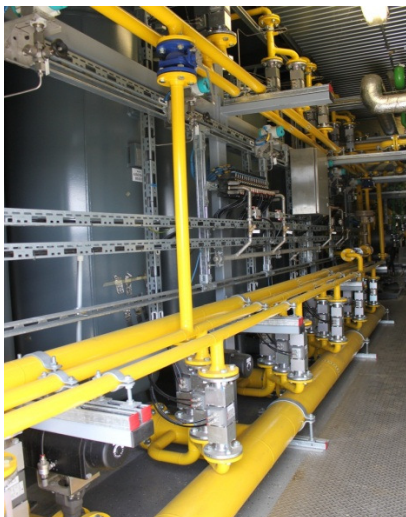
Figure 41: Pressure Swing Absorption (PSA) technology at Aiterhofen, Germany (Source: Rutz)
