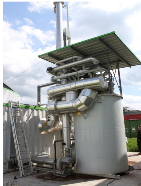
Figure 4: Low calorific value (LCV) burner of a biogas upgrading plant for digester heating in Aiterhofen, Germany (Source: Rutz)
